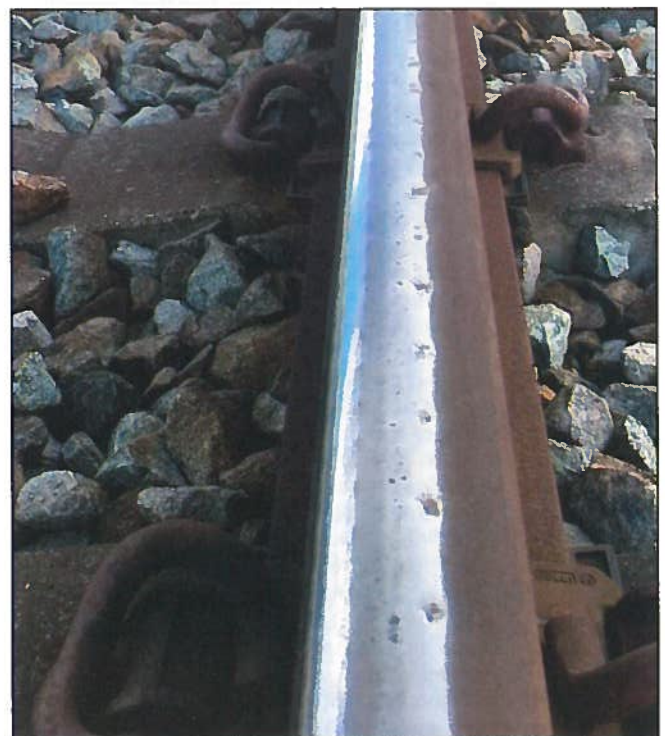
Fig. 4: Severe status of rail defect prior to grinding
