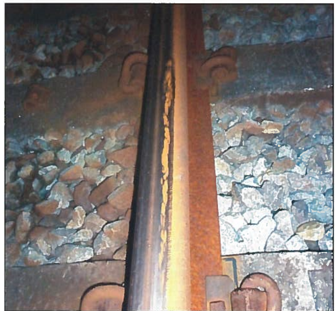
Fig. 1: Advanced centre-line spalling
