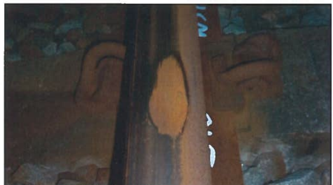
Fig. 2: Deep spalling in the rail head centre
